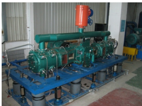
Fig.1 The reciprocating compressor
