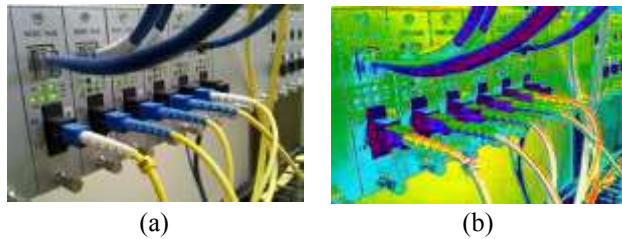
Fig. 7. Visual Inspection of optical Router-Switch cables reveals the existence of electrical anomalies (Sample 3) a) RGB regular image, b) Thermal Image
