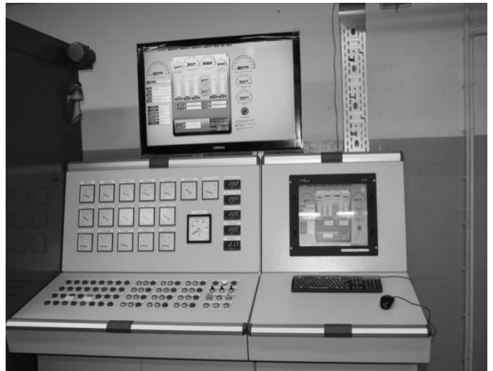
Fig. 2. General view of operating station EMOS
