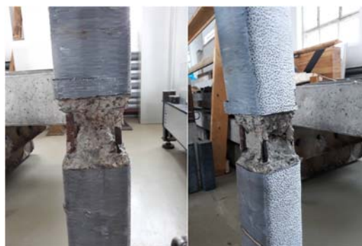
Fig.11. Stereo pair: two photos of a concrete bulk damaged in a building accident
