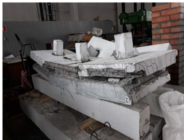
Fig.12. Ruins of the collapsed concrete floor, submitted for examination
