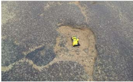
Fig.2. A picture of pothole in the road surface
