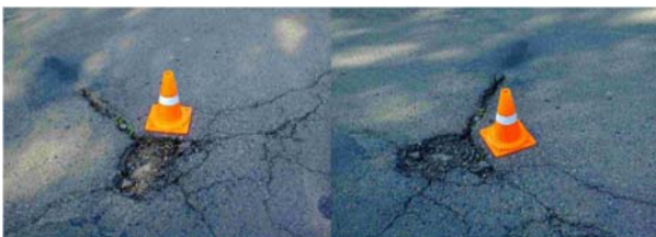
Fig.8. Stereo pair: road cone on the background of damaged road surface
