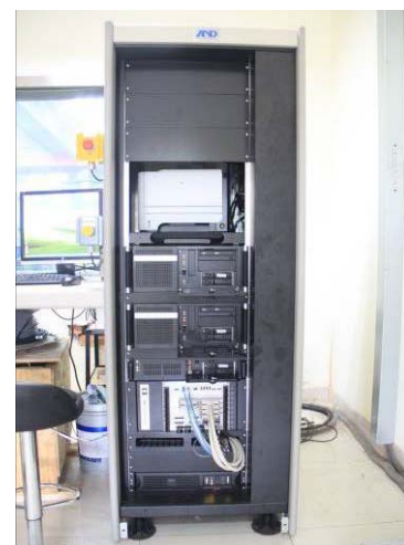
Fig. 13 The control cabinet of the DPS
