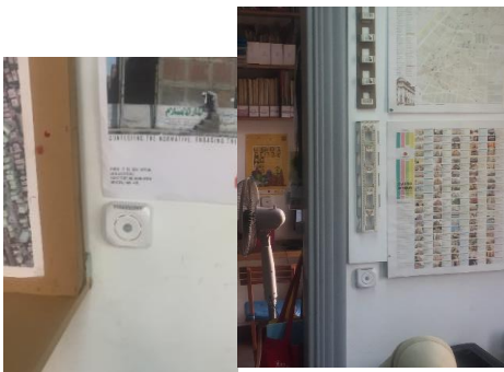
Fig4: Samples of the sensors installed
