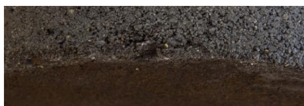
Fig.3 Typical detail of edge of concrete after 100 cycles of frost resistance
