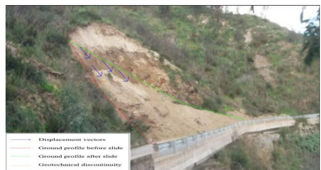
Figure 14 - Superposition of the displacements at break of the section aligned with the landslide. Example applied on the Reginella Landslide.
