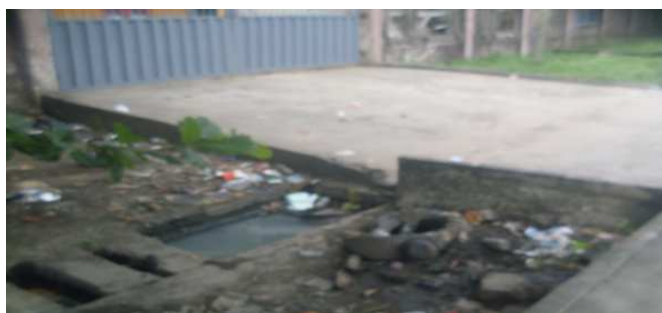
Fig 4: Poor drainage in off Bishop Oluwole Street, Victoria Island in Etio-osa
