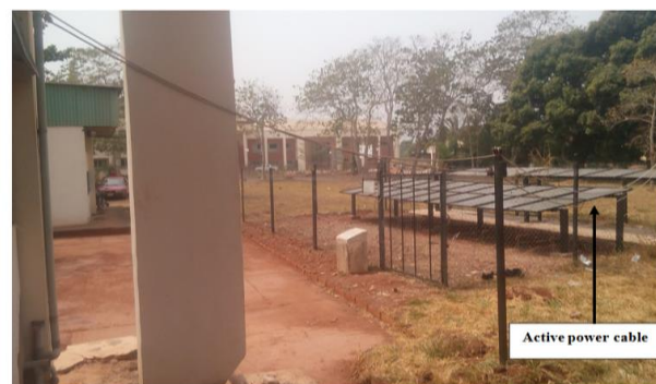
Fig. 22. Solar power Station.
